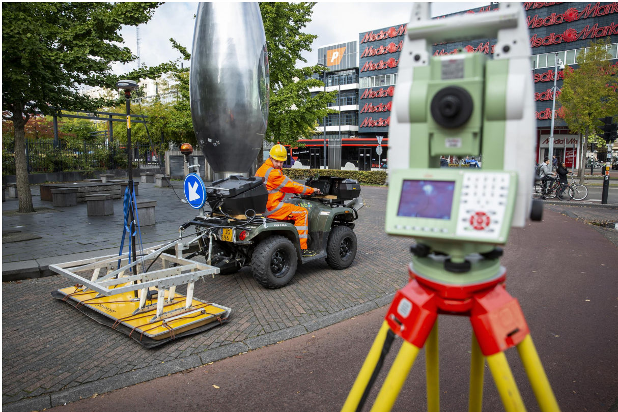
Our geophysics specialists examining the soil using modern measuring equipment and GPS-assisted geophysical surveying technique
