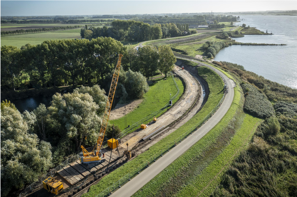
On our Gorinchem-Waardenburg (GoWa) dyke reinforcement project, we are using an electric wire crane. This 80-tonne crawler crane has a 37-metre boom (max. 58m) and operates completely emissions free
